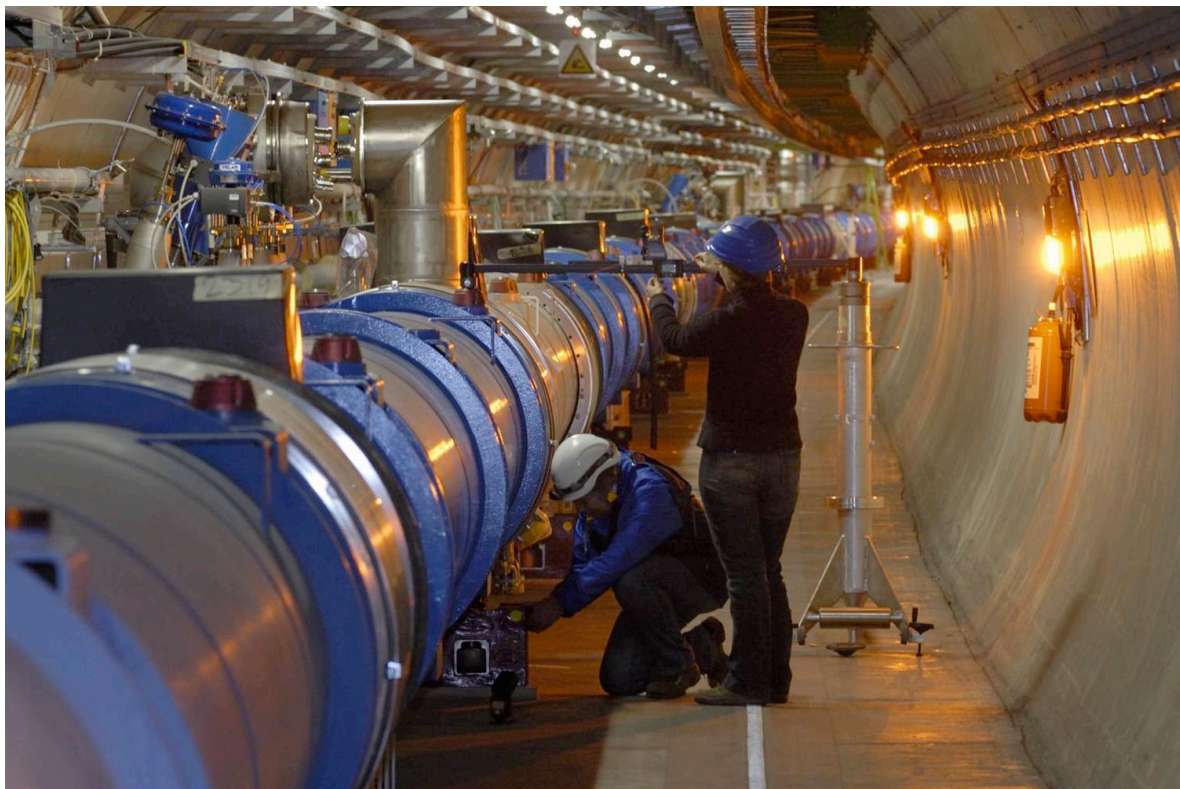
Picture of the installation of the dipole magnets and their connection to the cryogenic system in the LHC tunnel. (courtesy CERN)
