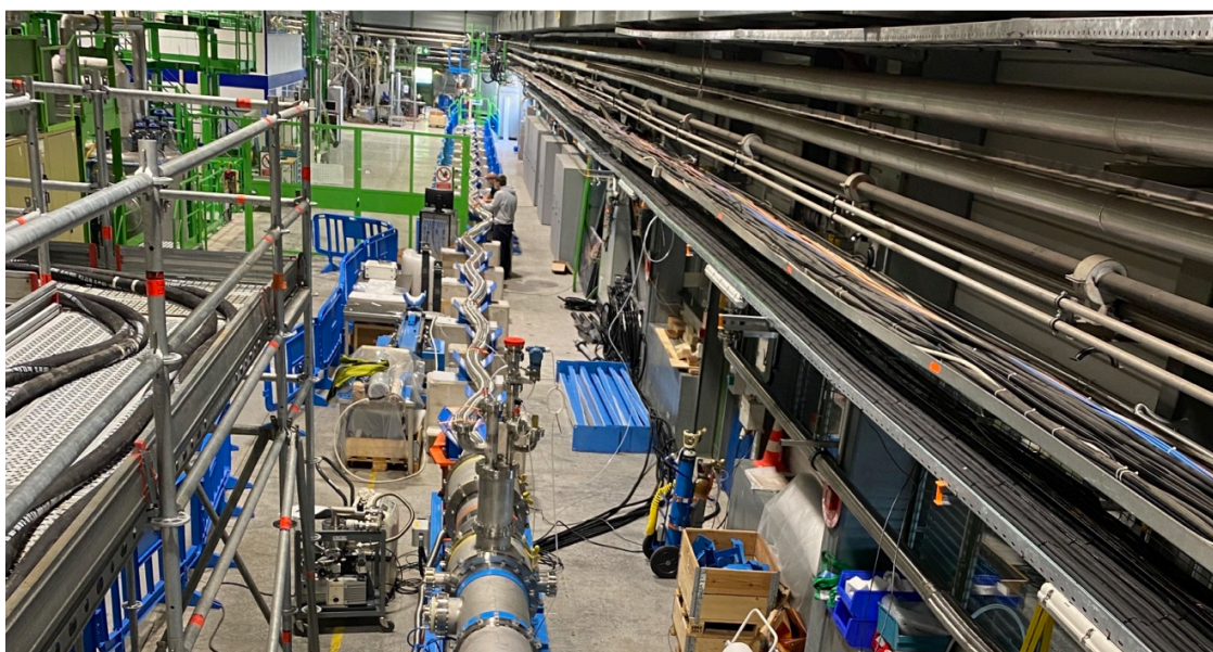
The 60-metre-long demonstrator of the superconducting electrical transmission lines for HL-LHC during testing in the SM18 hall at CERN.
